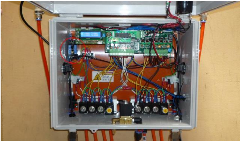
Figure 8. Control and Monitoring Unit with circuit breaker
